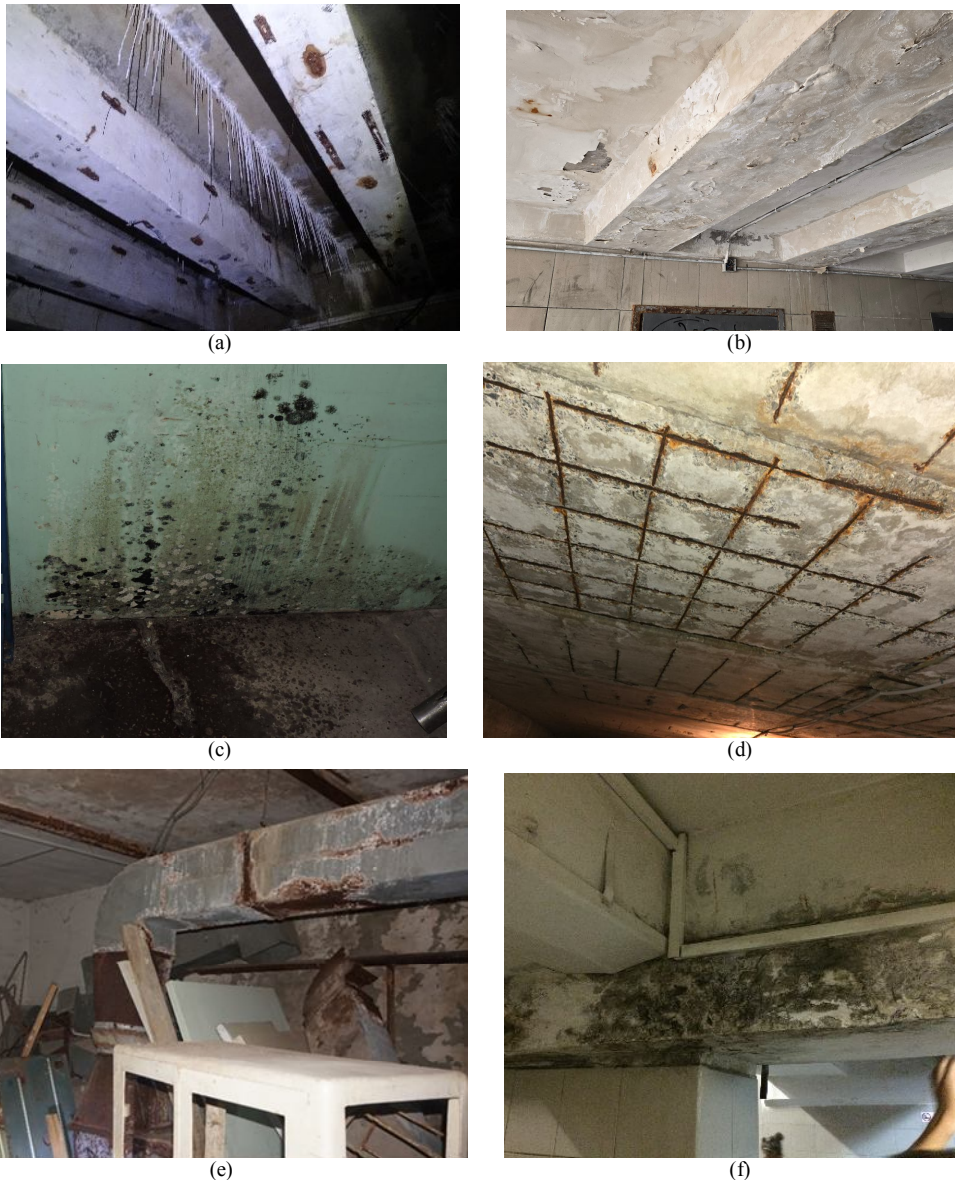
Fig. 1. Damage to structural elements of underground structures due to the action of moisture: (a), (b) – infiltration of water through the seams of structures; (c) – mold; (d) – corrosion of reinforcement; (e) – corrosion of engineering networks; (f) – damage to equipment and mold
