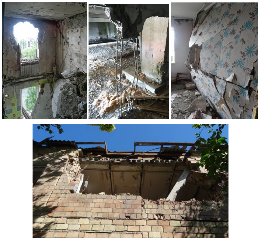
Fig. 4. Damage to structures due to the impact of projectiles from an MLRS, artillery, and tanks
