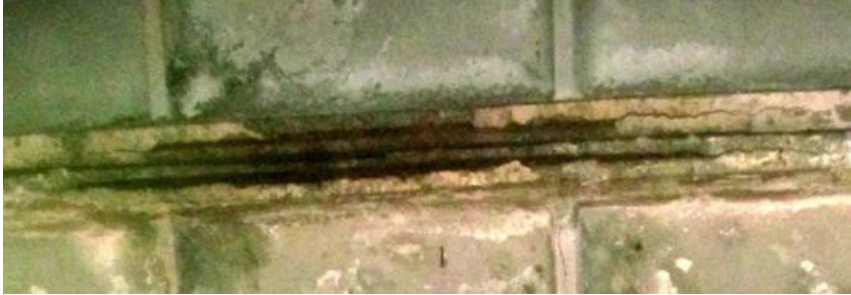
Fig. 1. Single cracks along the reinforcement on the edges of the ribbed floor slab
