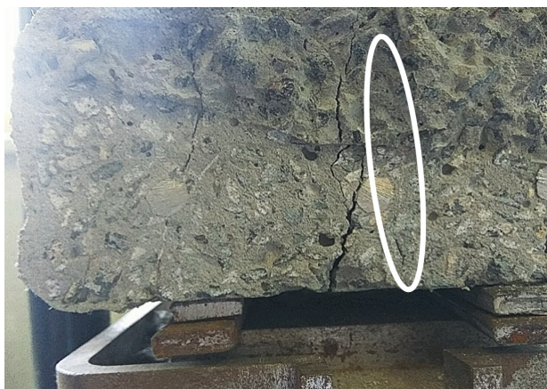
Fig. 6. New crack formed parallel to the glued (glued crack is marked)
