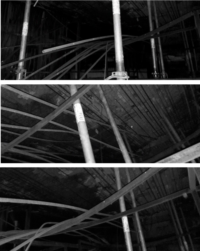
Fig. 8. Consequences of fire expose in «Auchan» store at «Sky Mall» shopping and entertainment center
